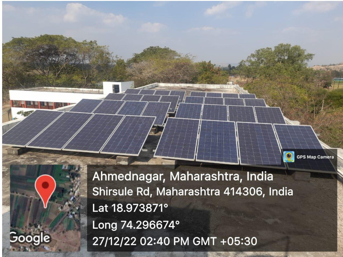
10 K. V. Capacity Solar plant fitted on top roof of A-Black Building
