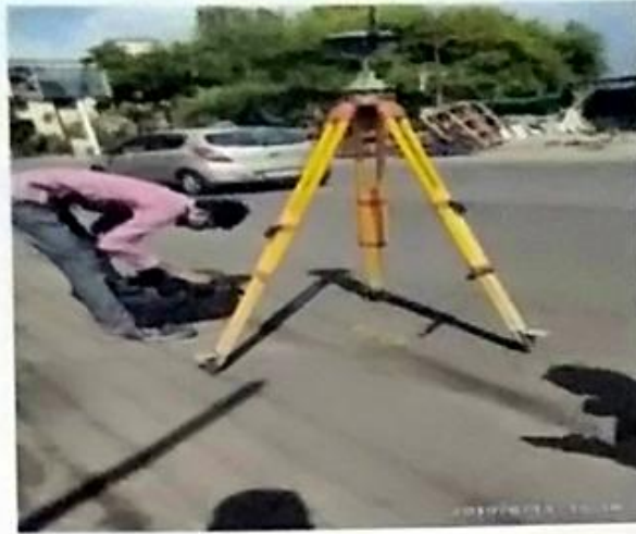
Shri Ajay Jadhav, Surveyor, Nighoj, Parner gives information about Total Station Survey with Field work.
