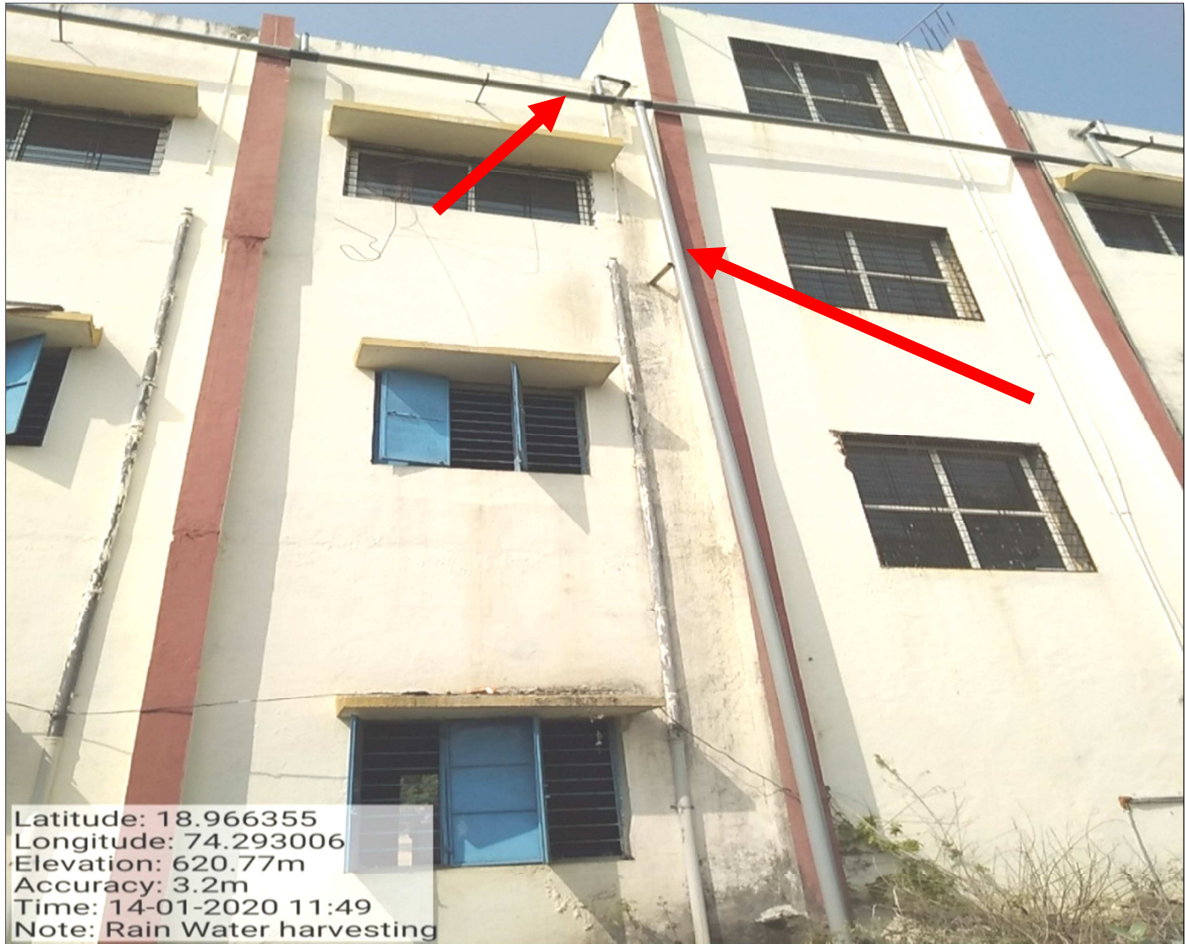
Photograph of Pipe Channel System for Rain Water Harvesting
