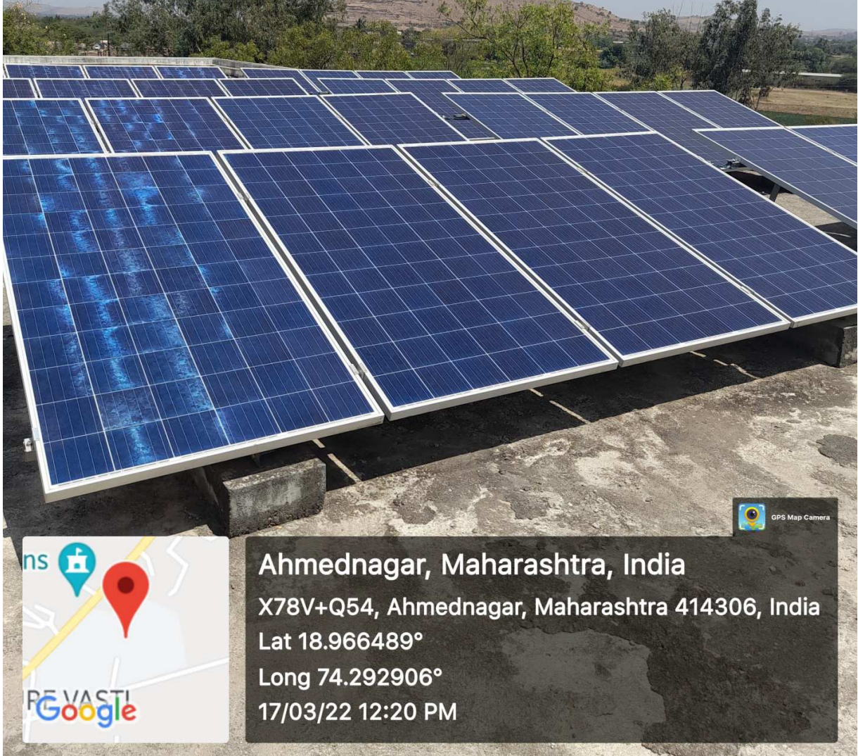
10 K. V. Capacity Solar plant fitted on top roof of A-Black Building
